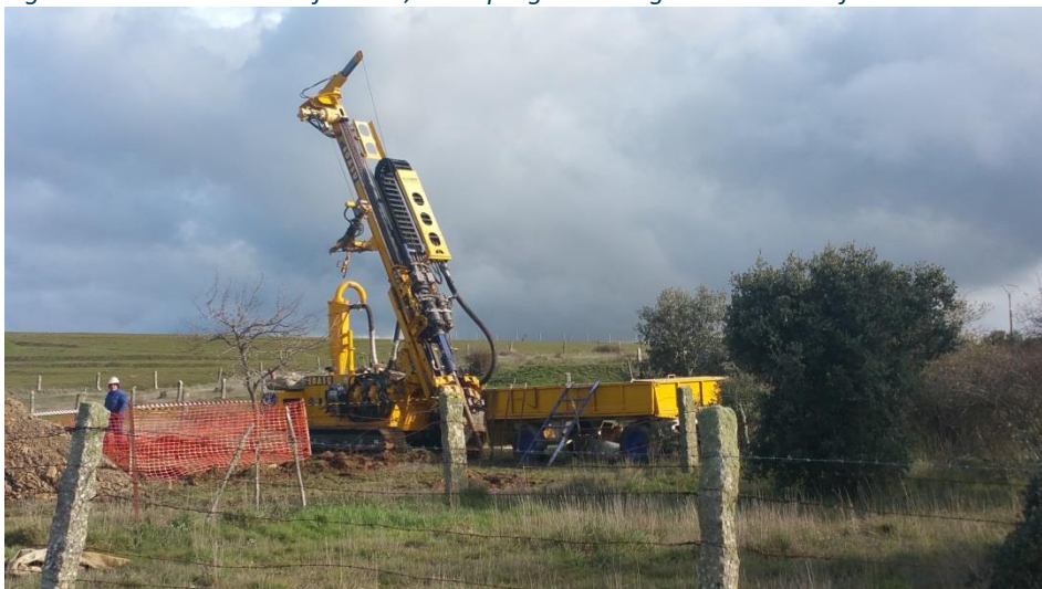
Figure 10: First drill hole of the 11,000m program being drilled north of Zona 7
